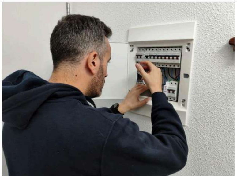
Figure 27: Shelly Pro installation in a user's electric board
