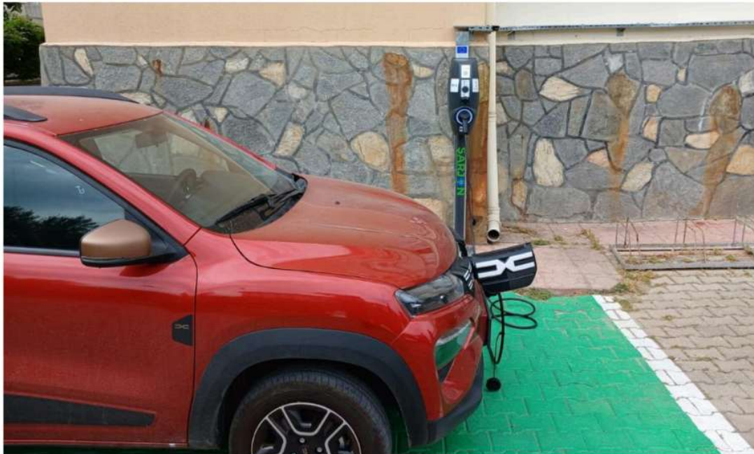
Figure 67: EV Charger while charging
