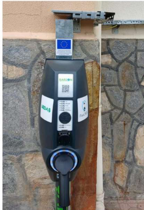
Figure 66: EV Charging Station
