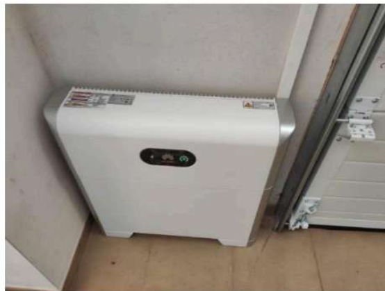
Figure 23: Battery - Spanish pilot
