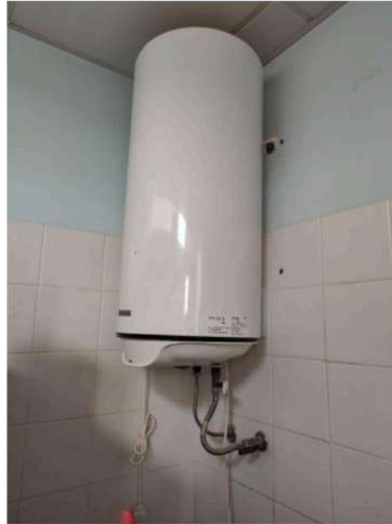
Figure 25: Flexible load: DHW tank - Spanish pilot
