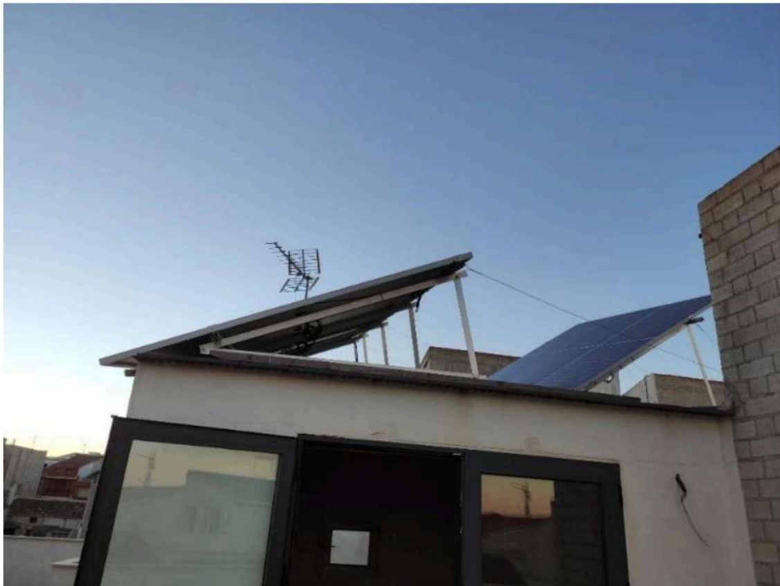
Figure 21: PV plant at municipality rooftop - Spanish pilot
