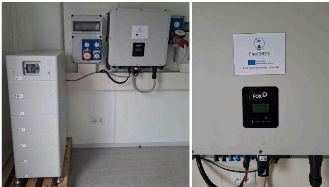
Figure 39: Small-scale battery of the Italian pilot
