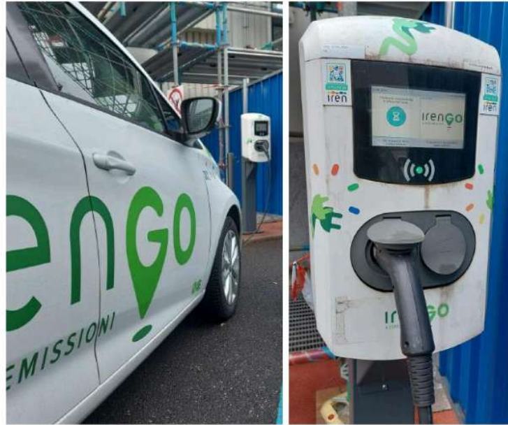
Figure 38: Example of EV charging station of the Italian pilot
