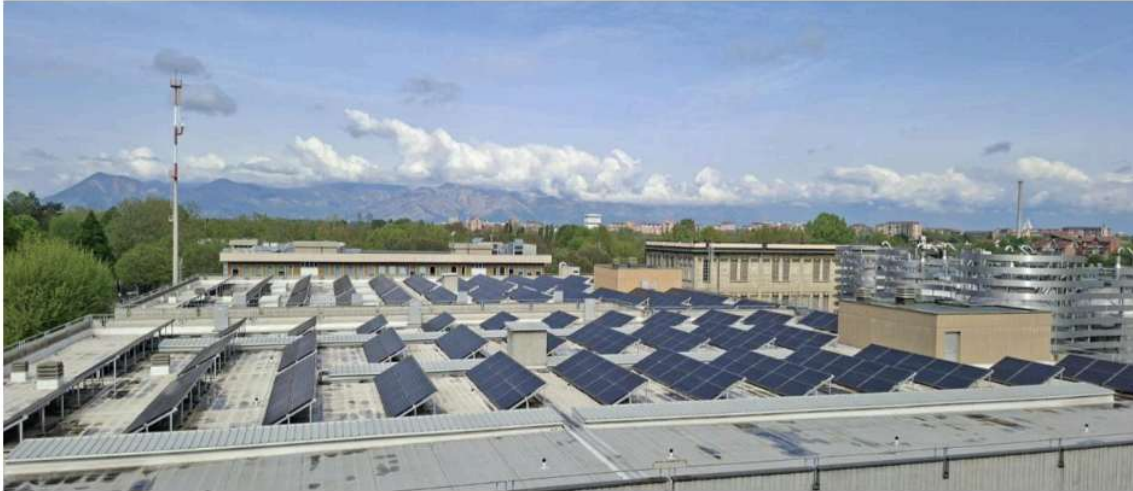
Figure 37: Rooftop PV array of the Italian pilot
