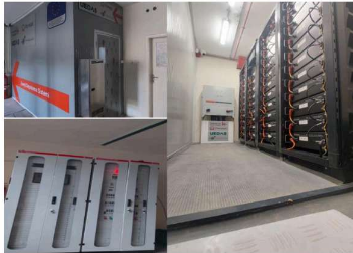
Figure 62: 100 kWh Battery Energy Storage System (BESS)
